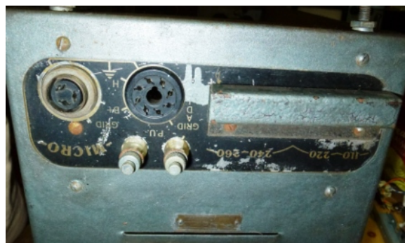
Older PA with hazardous terminals; hardened and crumbling rubberized wire insulation; &amp; optional DC powering with vibrator. Circa mid 1940's Australian Sound Systems A13.
